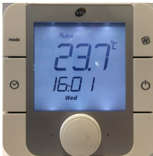
Figure 35 - Air Handling Unit in On mode
